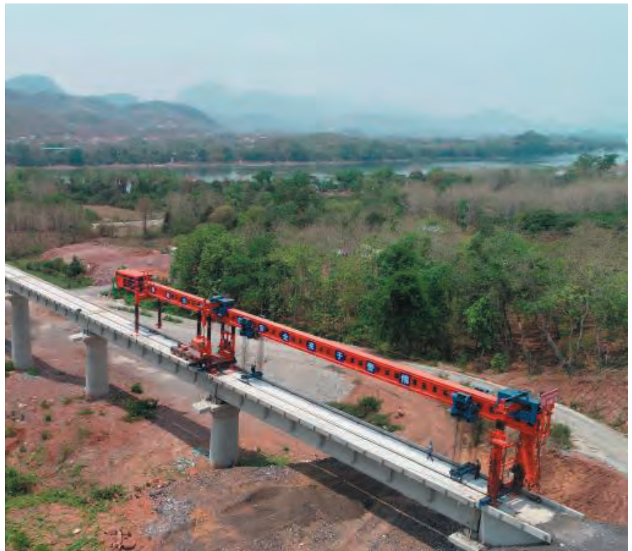
China-Laos Railway workers build the Luang Prabang cross-Mekong River Railway Bridge north of Vientiane, Laos, on April 23
