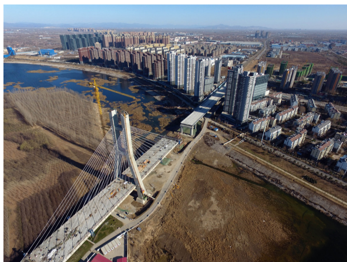
Chaobaihe Bridge, which will connect Beijing's Tongzhou District and Hebei's Yanjiao County, under construction on November 27, 2016 (XINHUA)
