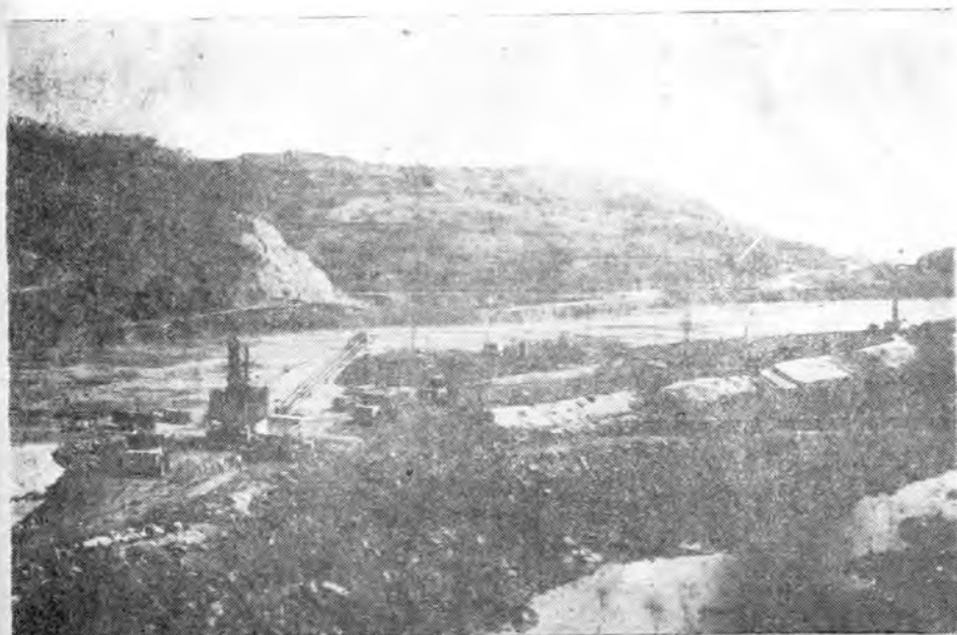
Building a reservoir in Cao Ngan district, Quang Nam — Da Nang province.
