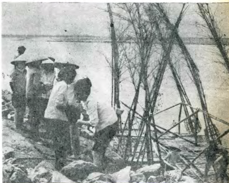
Repairing a section of the Red River dyke before the flood season.
