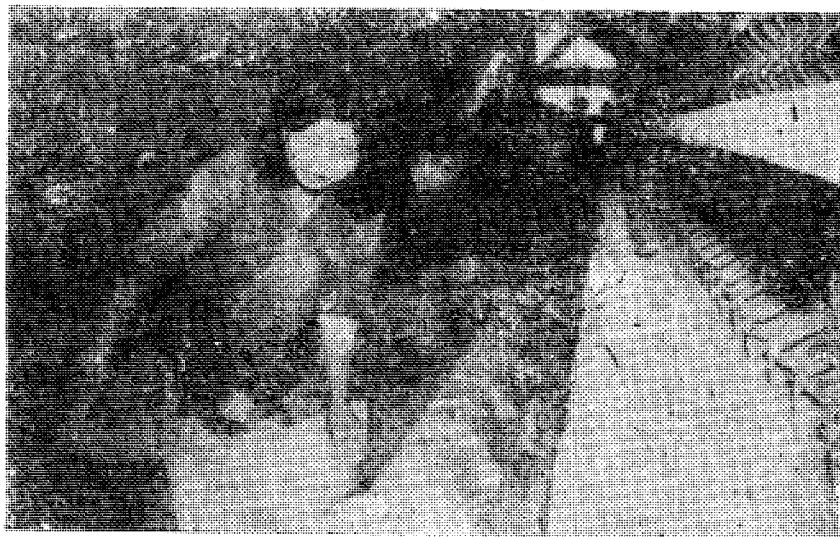
At the Hoang Thach cement factory: Lining a kiln with fire-resistant bricks.
