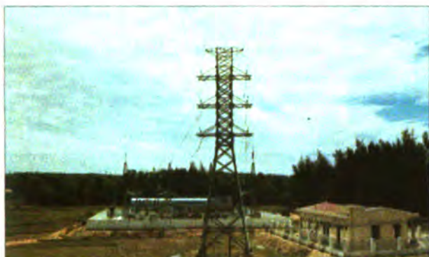
Trạm 110/22KV/25NIVA Trung tâm KCNDQ
