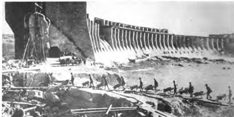
AT THE DNEIPER DAM —Work is going forward in rebuilding the great Dnieper Hydro Station, much of which was reduced to rubble during the war
