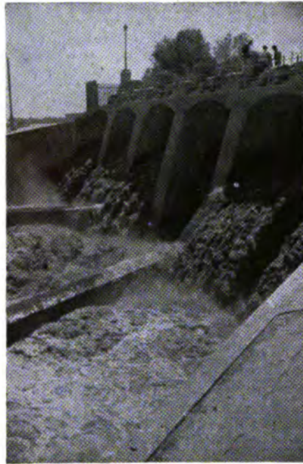
An extensive irrigation dam on the Tedzhenka River, one of the numerous works completed in the Turkmen Republic to facilitate agriculture
