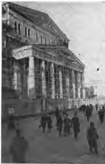
The Grand Opera and Ballet Theater damaged by a fascist bomb undergoes repairs
