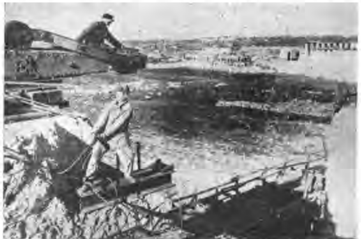
AT DNEIPER—Workmen begin the huge work of reconstructing Dnieper Dam, which during the war was seriously damaged
