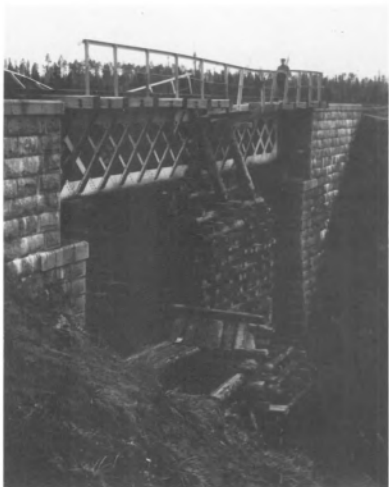
A bridge on the Archangel-Moscow Railroad. Both sides in the conflict were supplied by rail; Yank engineers repaired bridges as fast as the Bolsheviks burned them.
