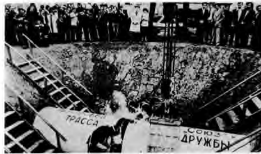
Welding the final joint of the international gas pipeline at the Soviet-Czechoslovak frontier.
