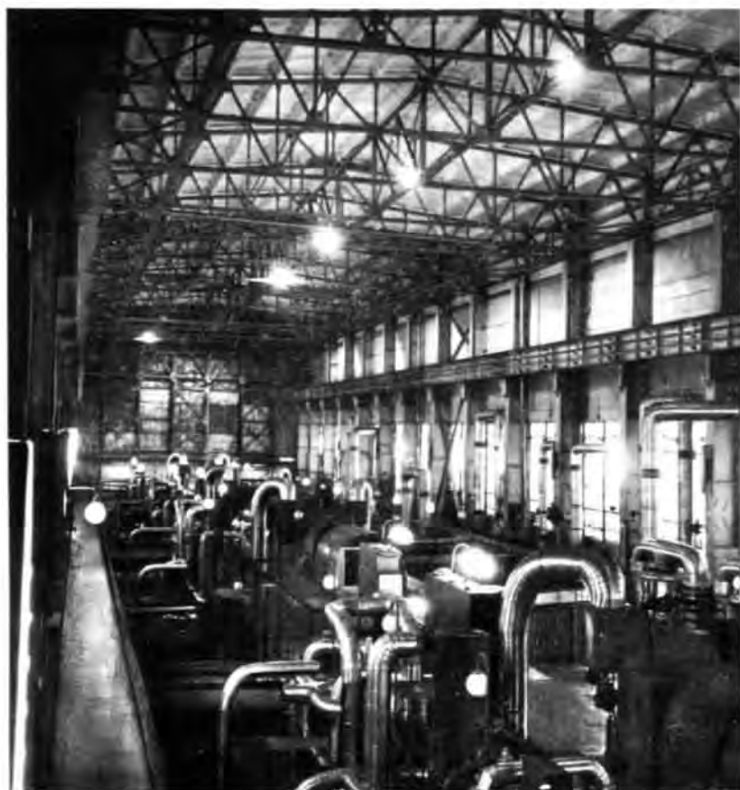
Soviet-made power generating units in the machine hall of the Darkhan thermal power station in Mongolia
