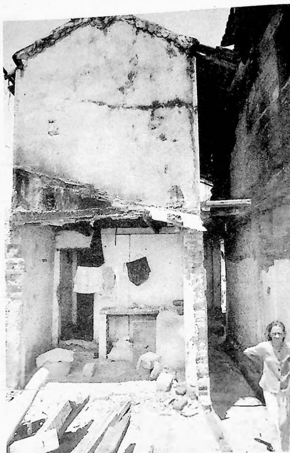
House damaged by tsunami, Galle.
