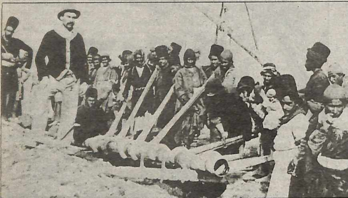
Arab workers lay oil pipe for the British prior to World War 1.
