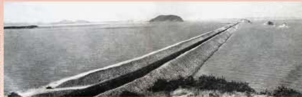
A long-distance conveyer belt has been laid at the Unnyul Mine
