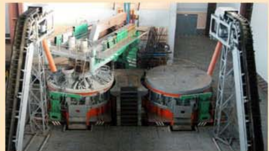
A double-body UHP electric arc furnace which uses domestic raw materials and electrodes
