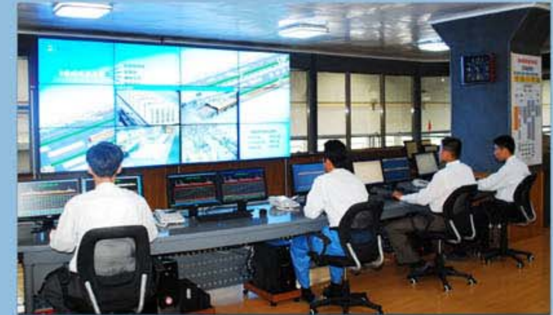
Second-stage general control room
