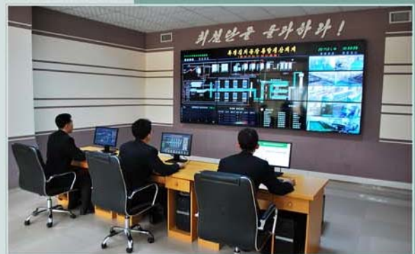
The general control room.
