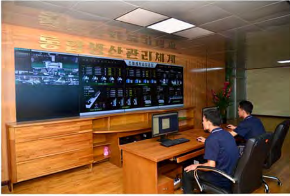
The integrated control room.
