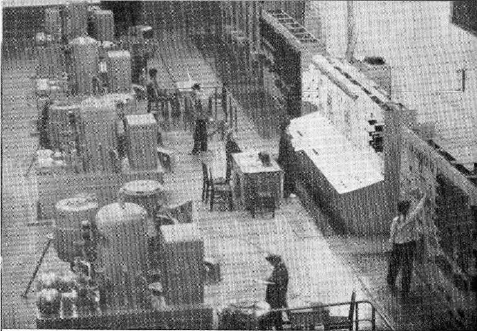
Control room of the Nachin Hydro-Electric Power Station.
