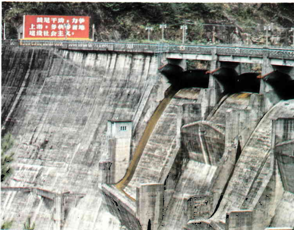
Commune members at Liang Kou built this dam to take advantage of the natural water flow in order to generate electricity. The sign at the top reads: "Go all out, aim high, to achieve greater, faster, better and more economical results in building socialism." (Photo: C. Kissinger)
