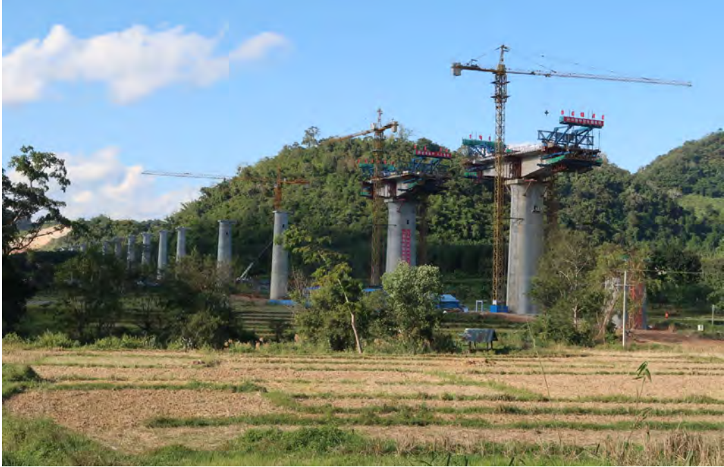
China–Laos Railway, project site of China Railway No. 5 Engineering Group, in Oudomxay province, Laos, 2020. PC: Jessica DiCarlo.
