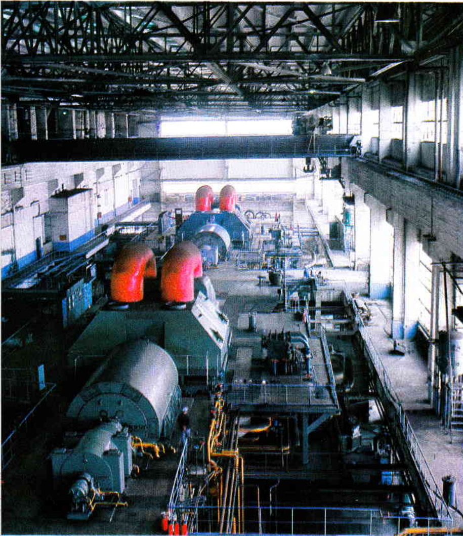
Motor room of Shentou mining power plant in Datong coal fields.
