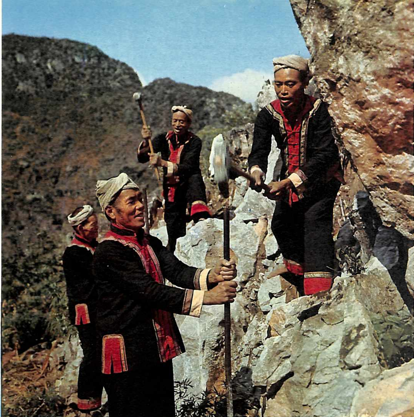
The "Foolish old men's field-building team" formed by four poor peasants of Yao nationality. In seven years on three mountainsides, they made three hectares of fields with a total of 110 terrace steps and 30 kilometers of stone embankments.
