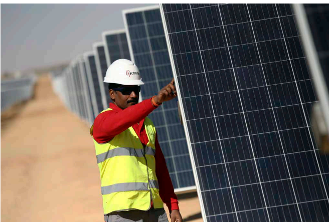
A man works on a Chinese-built photovoltaic power project in Aswan, Egypt, on March 18
