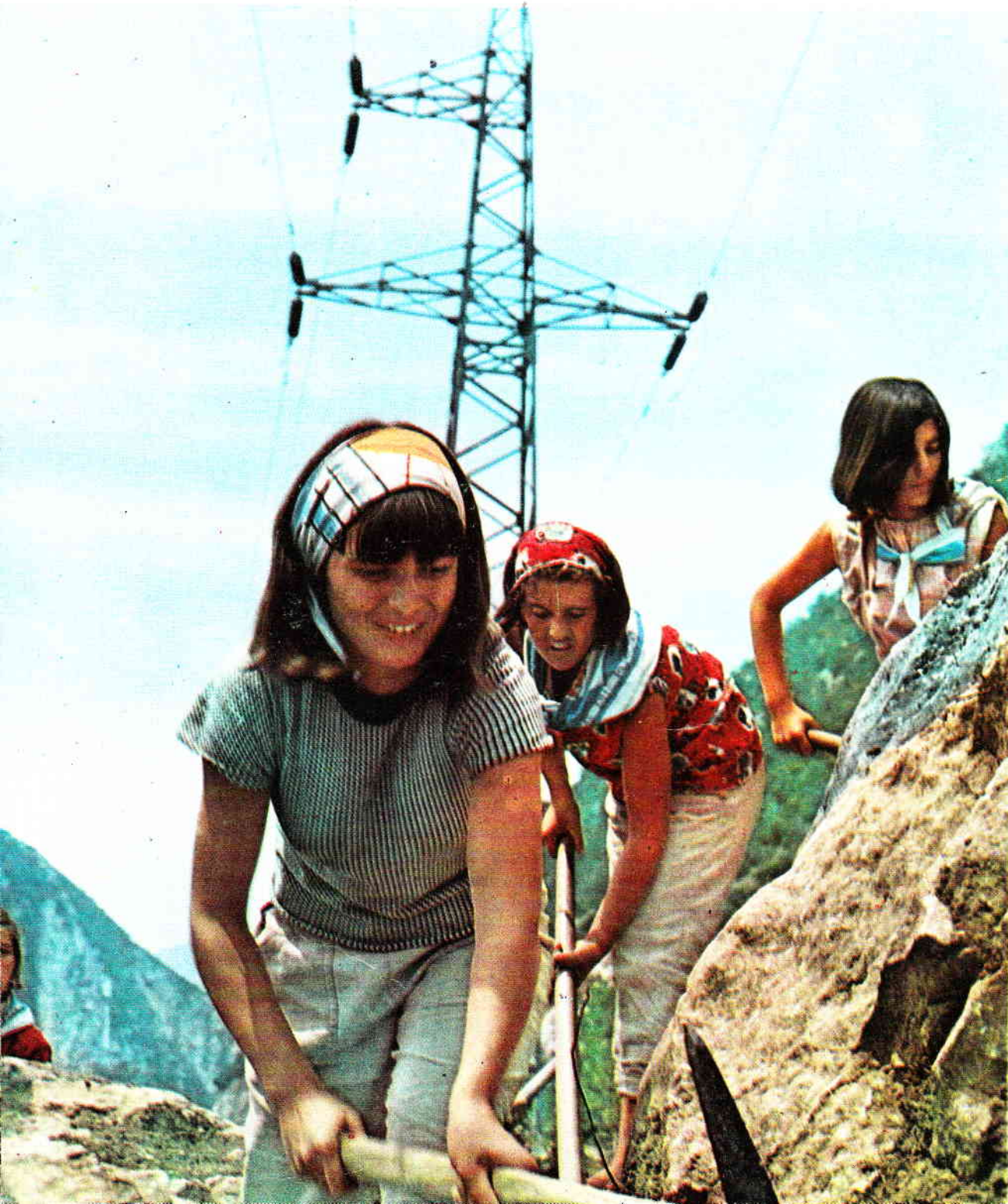
Our young men and young women study and work, they take active part in the building of the homeland. In the photo: A snapshot of the work of a group of youths volunteering in the construction of the Fier-Ballsh railway.
